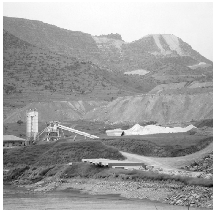
Building-work resumes at Ilisu dam construction site. Photo by Initiative to Keep Hasankeyf Alive.
