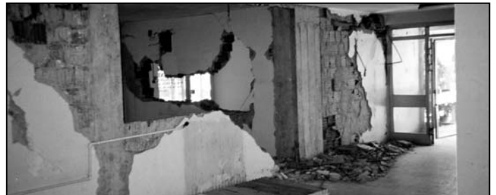
The building which houses the Mayor's office in Bingöl. There have been no repairs since the earthquake, June 2003
