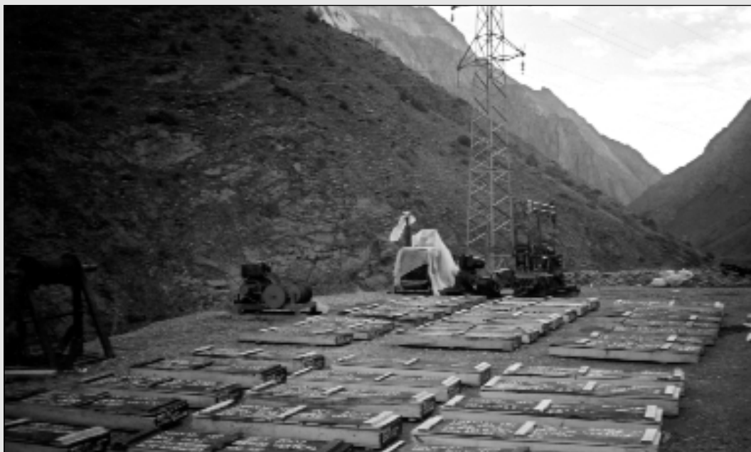
The KHRP delegation found preliminary drilling at one proposed site for the Hakkari Dam
