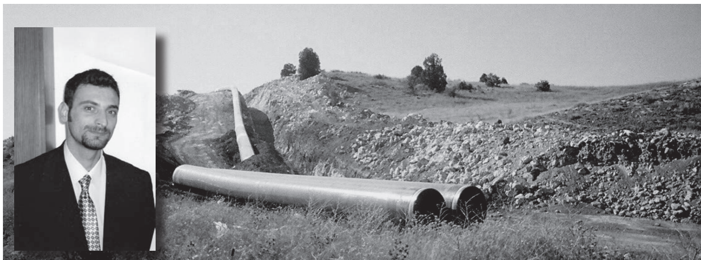
ABOVE: Construction of the controversial BTC pipeline, Turkey section INSERT: Ferhat Kaya, a human rights defender who believes his arrest and ill-treatment in detention were directly connected to his work regarding the BTC pipeline
