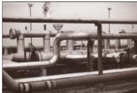
BP's Central Processing Facility, Tauramena, oil from which flows into the OCENSA pipeline (Michael Gillard)
