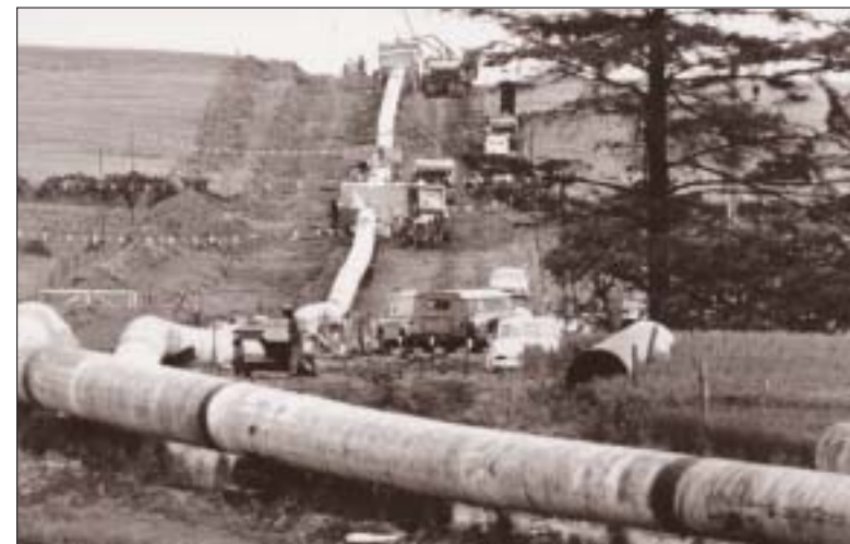
Construction of the onshore section of FPS, just south of Stonehaven, northeast Scotland, July 1973 (Press and Journal: Aberdeen)
