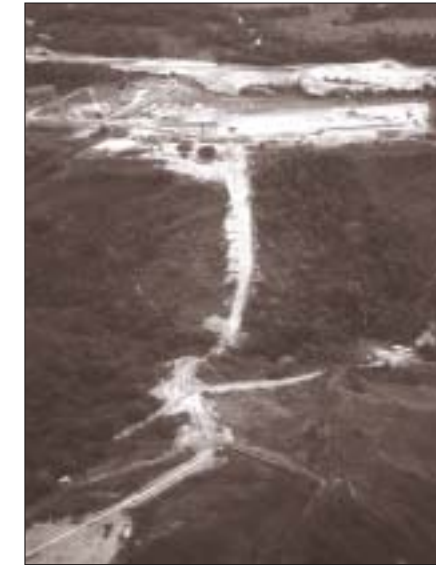
Construction of the Central Processing Facility (which feeds OCENSA pipeline) and pipeline from Cusiana-Cupiagua oilfields, Tauramena, March 1997 (Michael Gillard)
